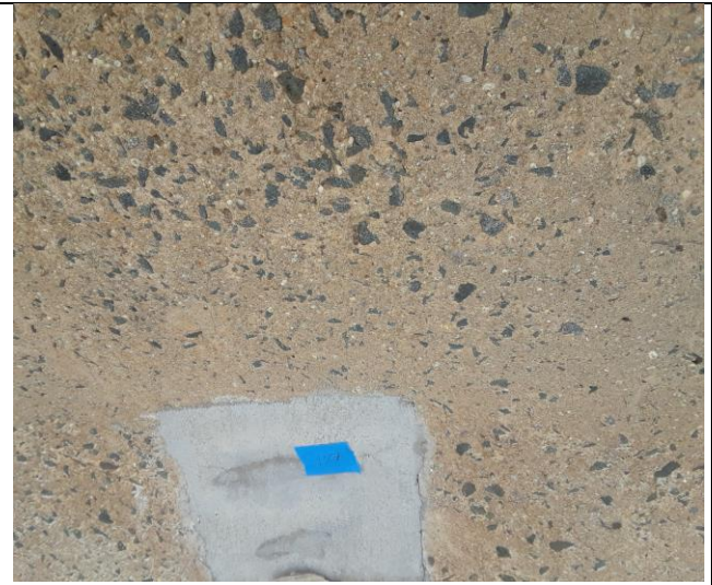
Picture showing mark deficiency grout pocket on the PCC Barrier
