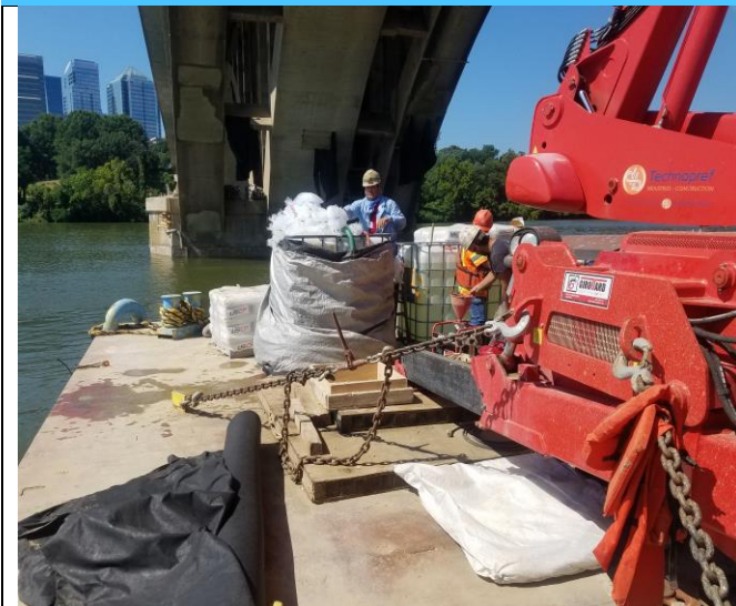
Technopref placing ice into water tank for shotcrete mixing to reduce conc temperature
