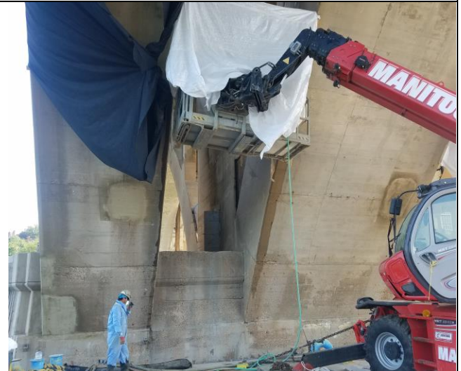
Ward & Assoc wet shotcrete contained patch at Span E Bay 2 Diaphragm close to Pier 3
