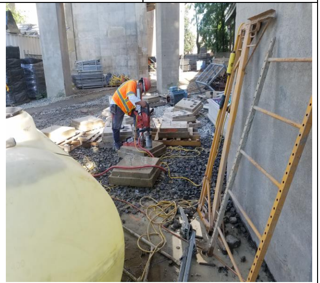
Technopref core drilling shotcrete test panel for sample for Lab on the staging area
