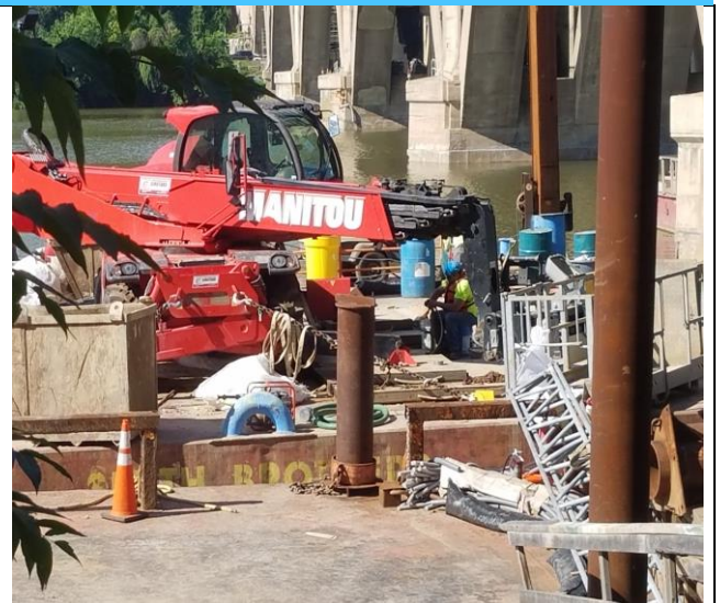
Technopref 007 with Manitou spudded at Shore with Manitou down due to Electrical Problem
