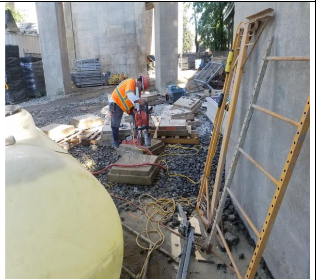
Technopref core drilling shotcrete test panel for sample for Lab on the staging area
