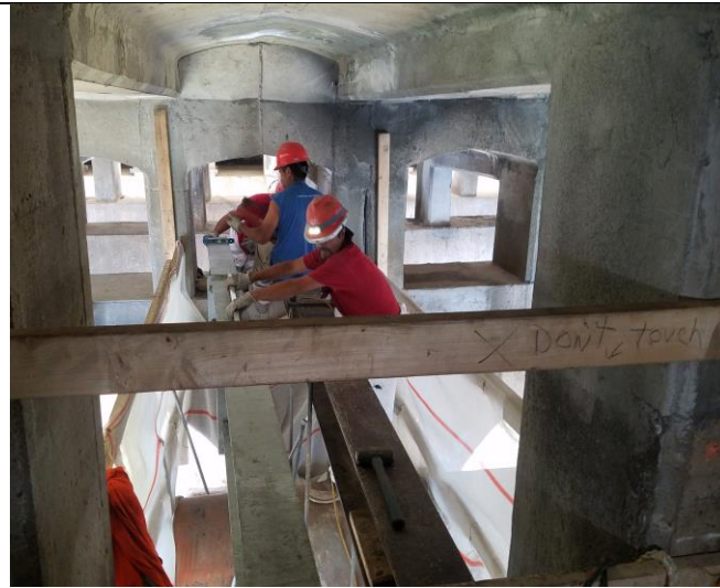
Technopref in West Gallery at Span D in process replacing DC Water 30 inch Main Support Beam
