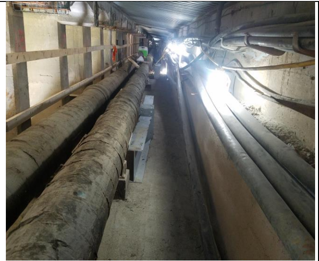
Technopref in West Gallery at Span D in process replacing DC Water 30 inch Main Support Beam
