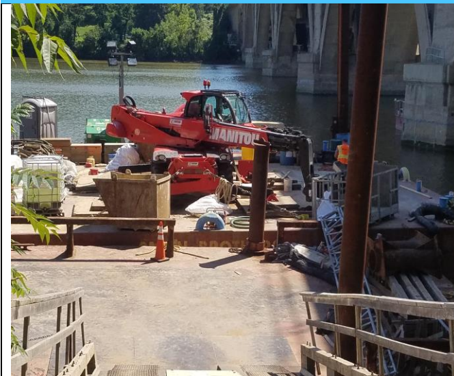
Technopref 007 with Manitou spudded at Shore with Manitou down due to Electrical Problem
