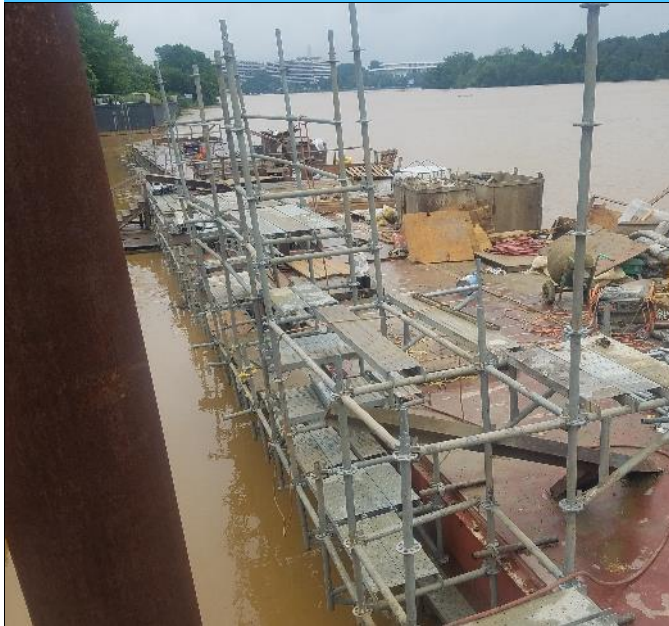
Barges spudded at shore as Key Bridge and Potomac River flood condition at high tide
