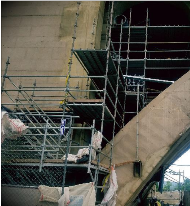
Rosslyn Abutment E Elev at Span H Row EE dismantling scaffolding & spall for repair
