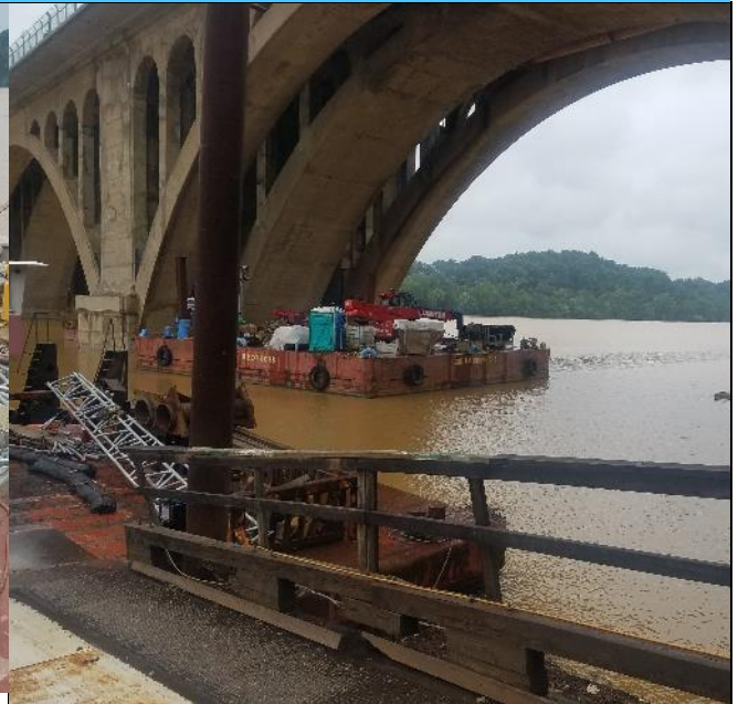
Barges spudded at shore as Key Bridge and Potomac River flood condition at high tide. Also square barge spudded at Span C
