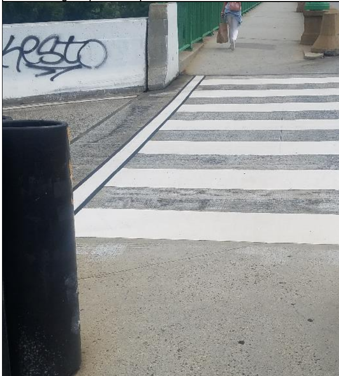
New Pavement Marking Crossing East Ramp exit on Key Bridge recently installed
