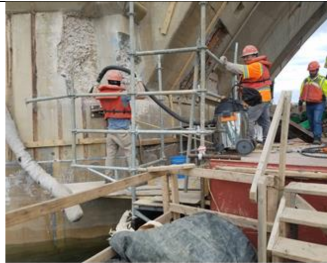
Concrete repair and saw cutting at Pier 2 base and the use of vacuum to clean debris.
