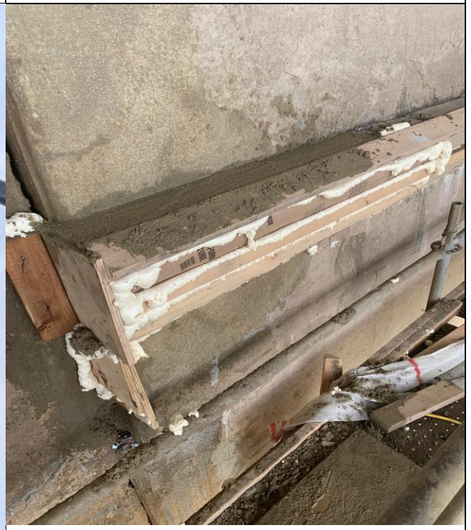
Form and pour for architectural fascia located at Rosslyn Abutment West Level 1
