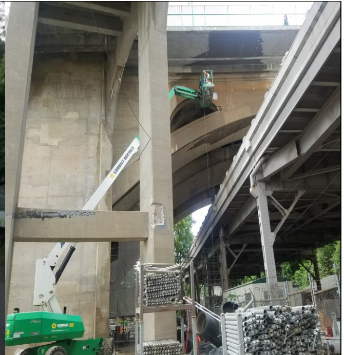
Power washing concrete portion of the Key Bridge on Span B East Fascia
