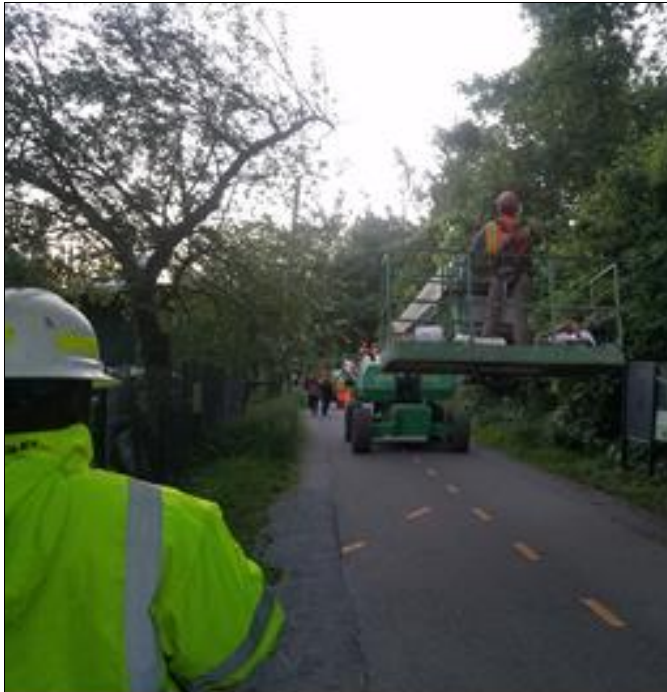
Contractor mobilized manlift to C&O Canal tow-path through the Capital Crescent Trail (CCT) up to the Foundry Branch stairs and ramp, then on to the canal towpath and travel down to the Key Bridge construction site
