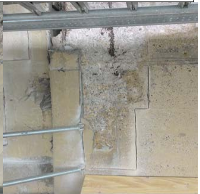
Fibrwrap demolition of marked concrete repair area on N Abut west side level 1 SW corner. (unfinished work)
