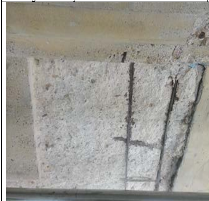
Fibrwrap demolition of marked concrete repair area on N Abut westside level 1 SW corner.(unfinished work)
