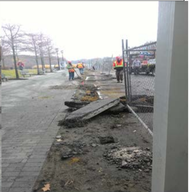
Removing existing fence for the NPS 8 ft. tall wood lattice and chain link fence
