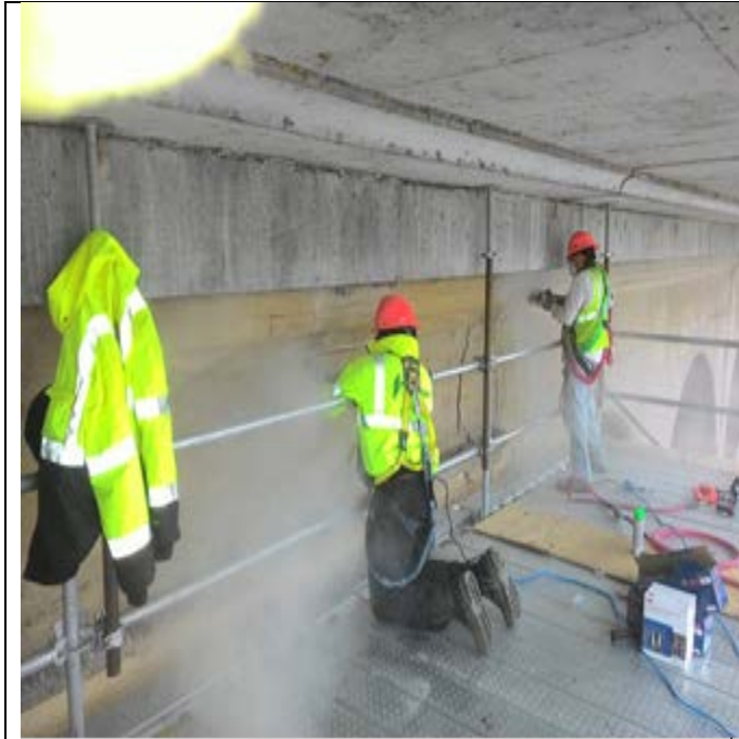
Fibrwrap saw cutting at scaffold level 1 for repairs on West of North Abutment
