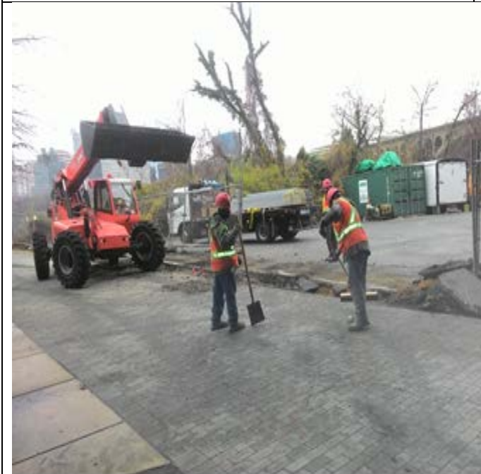
Removing existing fence for the NPS 8 ft. tall wood lattice and chain link fence
