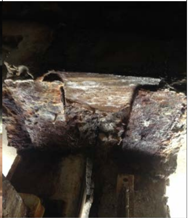
Floor beam end current condition.
