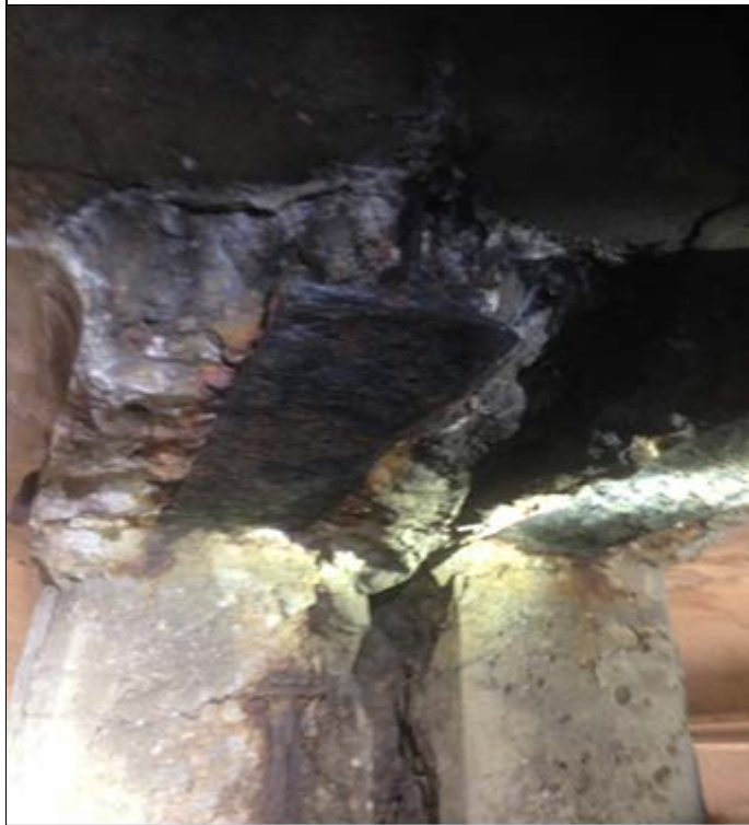
Floor beam end current condition.
