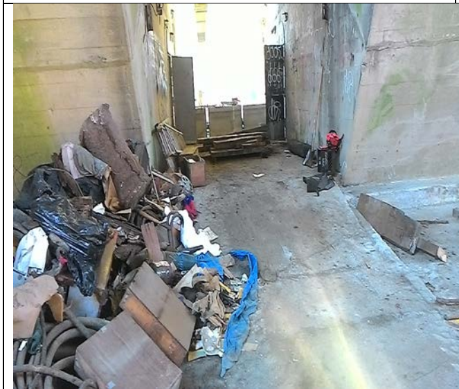
Debris from the chambers at North abutment
